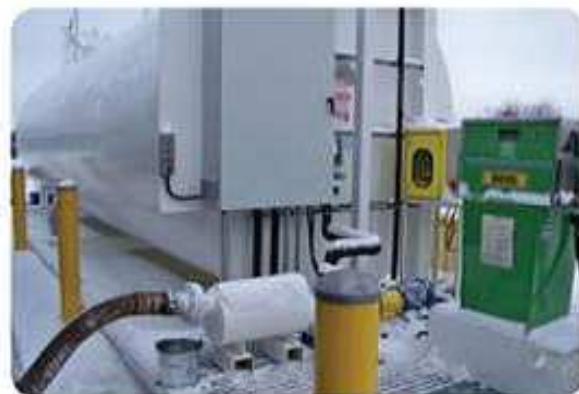
Typical above ground fueling tank receiving a delivery
