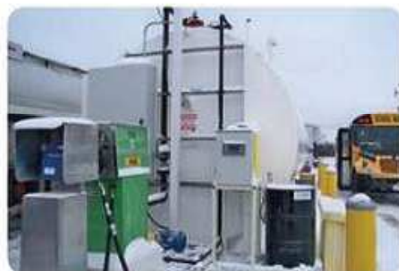
Typical above ground storage tank with Envirox dosing equipment
